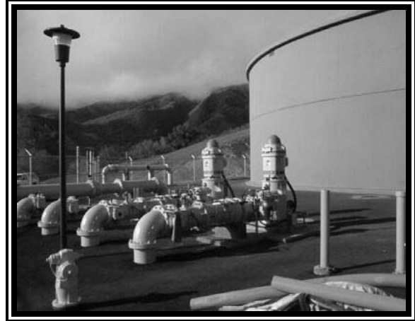
Photo: Example of a project that could be included in the CIP, storage facility installations
