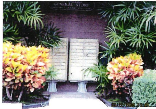
Centralized equipment at Shopping Mall
