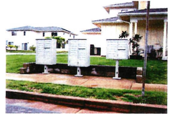
Centralized equipment installed by Developer
